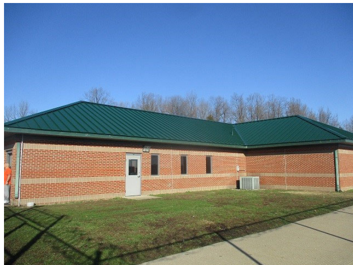
Pictured to the right: New metal roof on minimum security housing unit.
