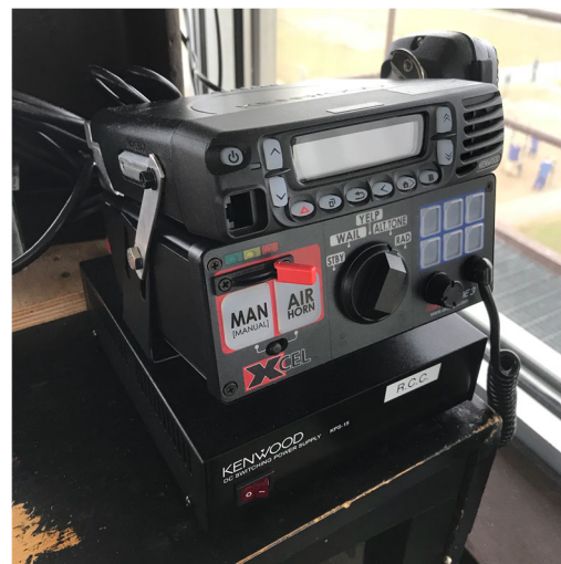
Pictured below: Yard compliance siren.
