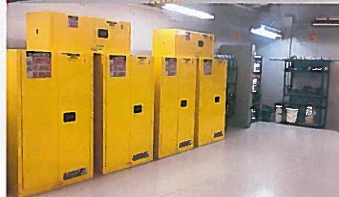
Pictured at the bottom left is the Caustic Toxic Room that was noted during the ACA Audit.
