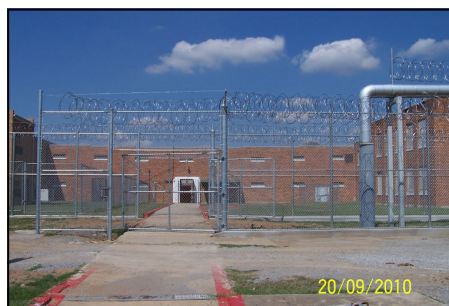
New interior fencing at Northpoint separates the inmates from the construction site
