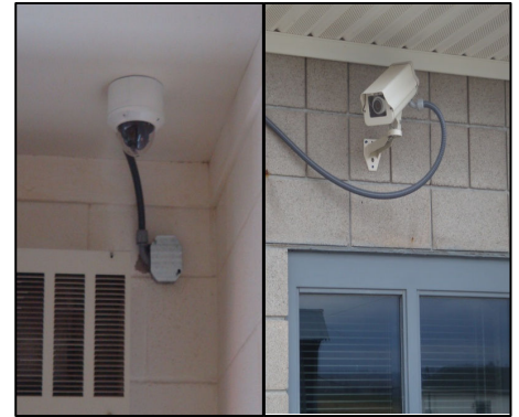
Minimum security unit security camera enhancements
