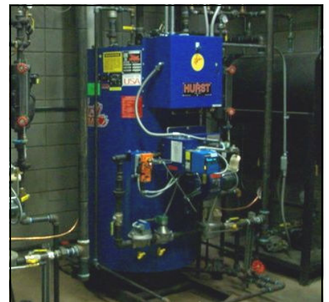
Gas Fired Steam Boilers for Kitchen Area.
