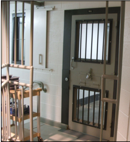
Replaced walk door windows in SMU with lexon and installed security bars.
